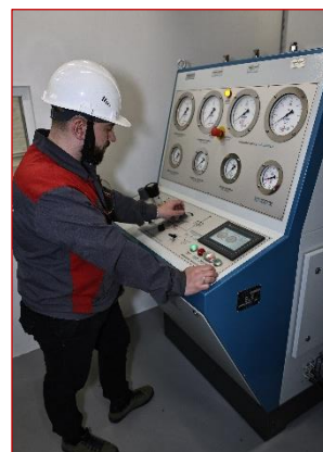
A pneumatic hydroelectric power station for hydraulic and pneumatic testing.
