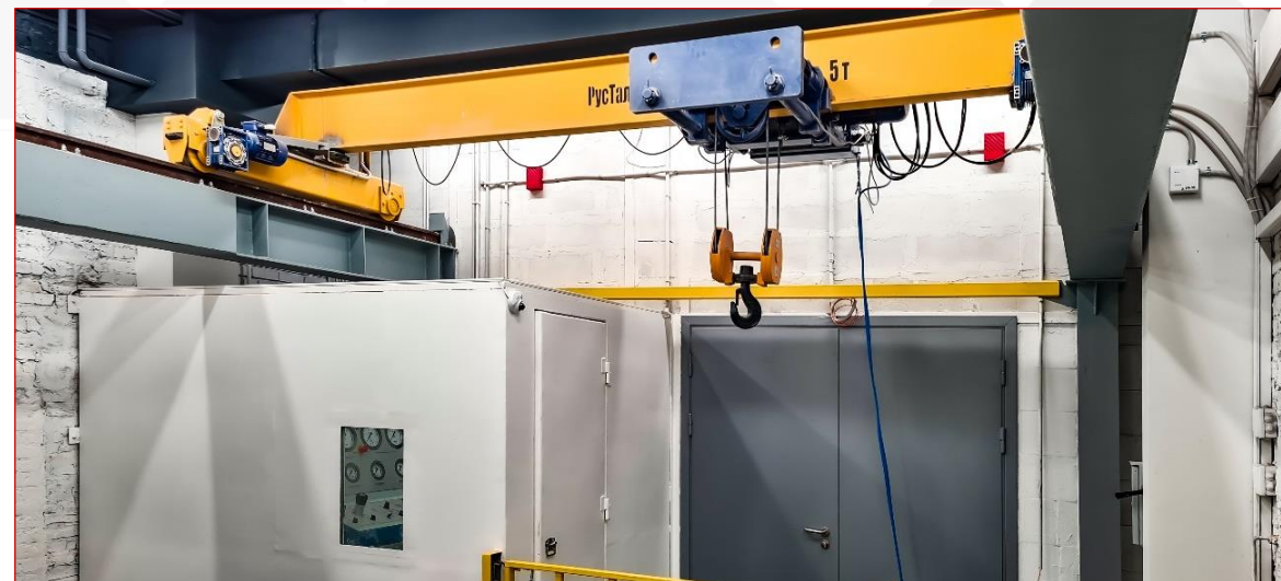
Single-girder overhead crane.
